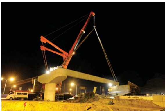
Night-time launch of the 40m beams, belies the complexity & meticulous preparation behind this apparently simple operation.
