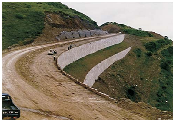
Construction Of The Large Reinforced Earth Retaining Wall On Tutor Ndamase Pass
