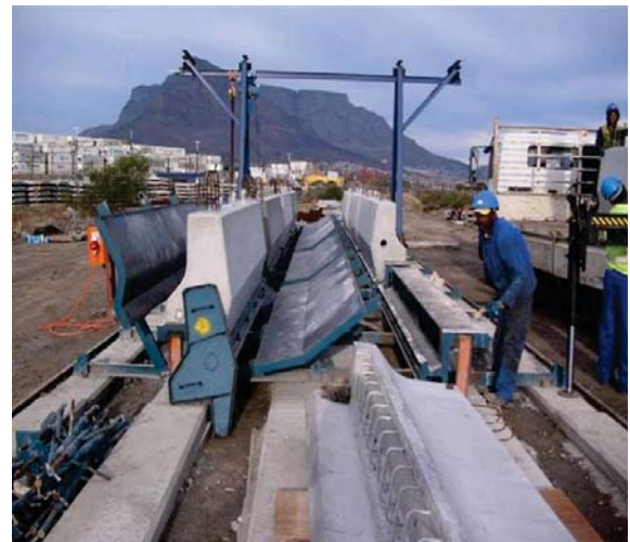
Innovative precast balustrades with linking system, essential to delivery on schedule
